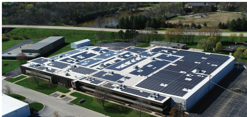
Martin Automatic's new roof with solar panels
